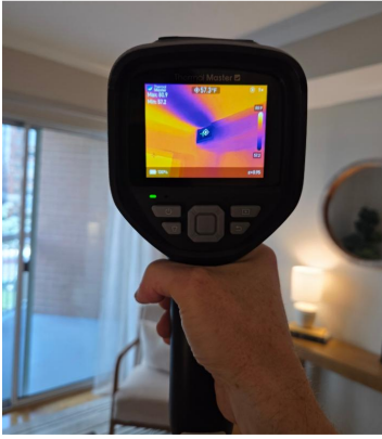
Register in Living Room showing adequate cold air temperature from AC Unit.
